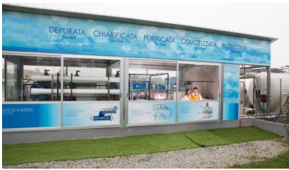
Reclaim installation, Settimo factory, Italy
