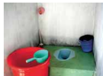
Typical pour-flush toilet connected to a septic tank
